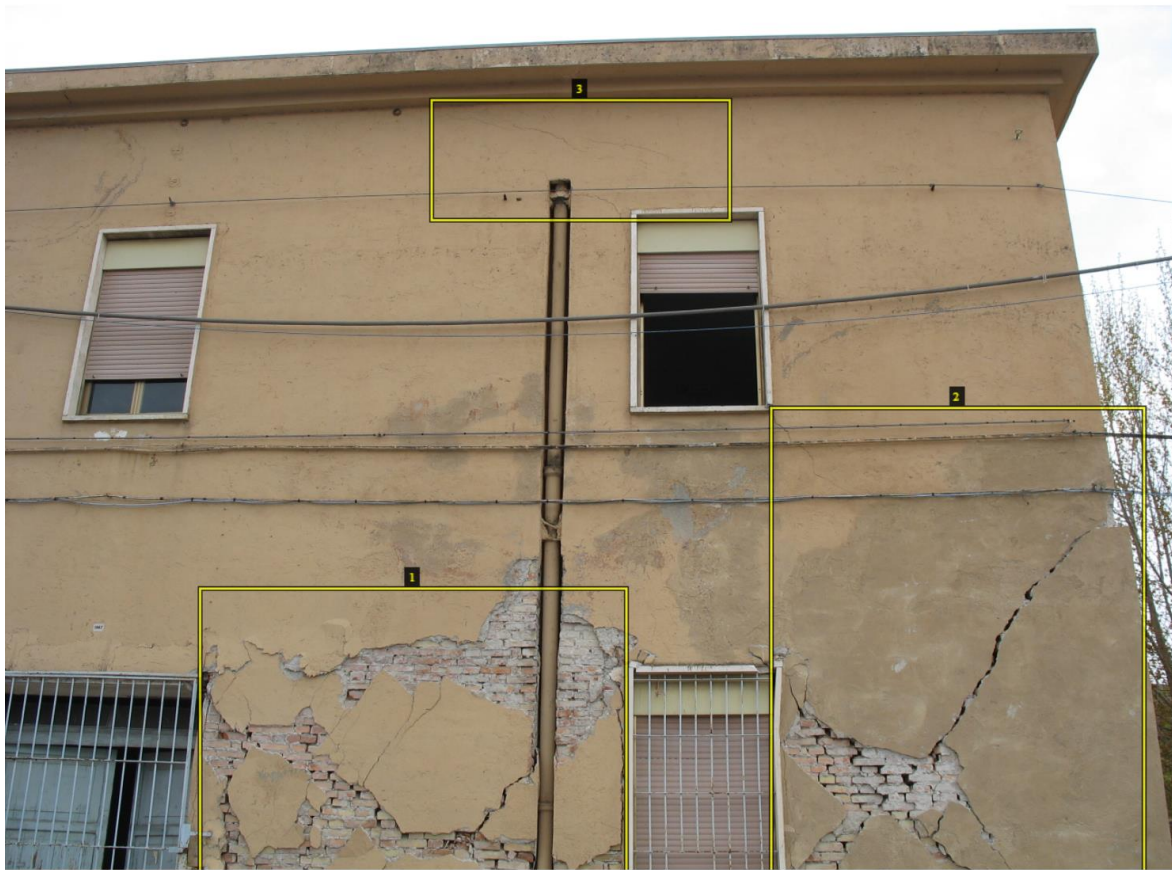
Figure 36: Example of an annotated image belonging to EUCENTRE'S dataset (L'Aquila 2009 event, shear damage on unreinforced masonry piers and spandrels)
